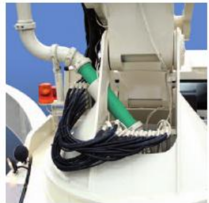
The orderly placement of hydraulic and pipe lines allow good accessibility to the turret.
