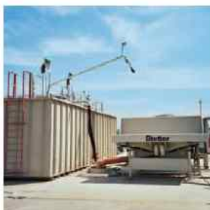
Aboveground design with double container for the temporary storage of waste water, recommended for rocky foundations or mobile use.
