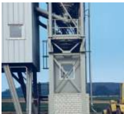
The raised control container with MC control system and high-voltage section allows free sight to the discharge hopper of the mixer.
