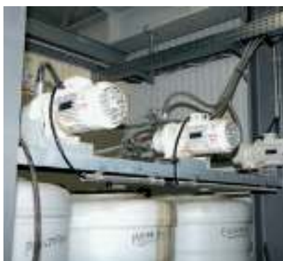
The plastic tanks for storing of the admixtures are filled from level \pm 0 . All fill lines are centrally combined.
