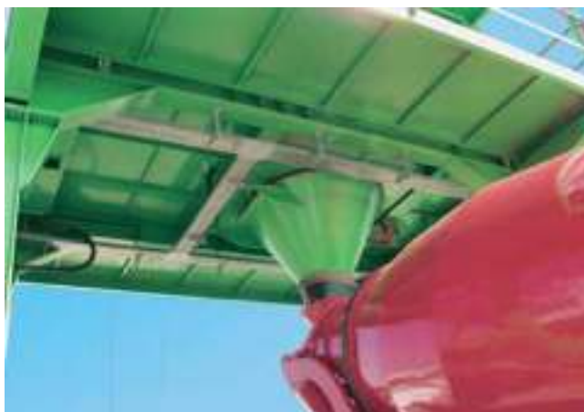
The mixer discharge for filling truck mixers.
