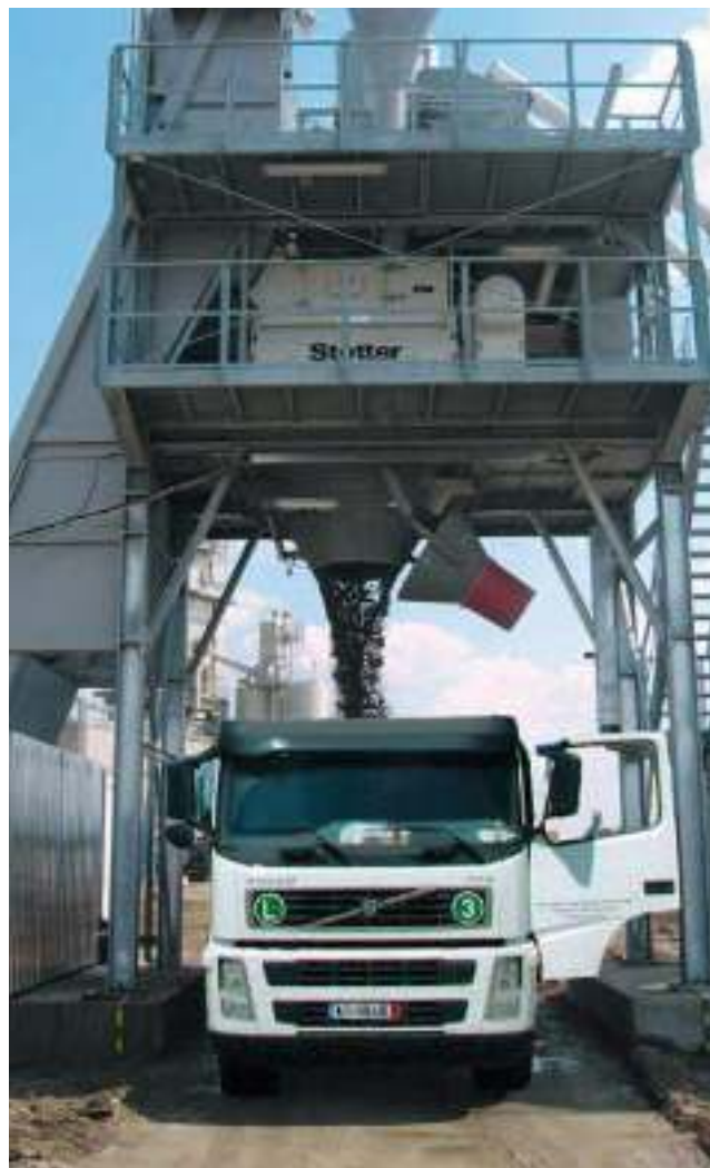
Discharge onto open truck.
