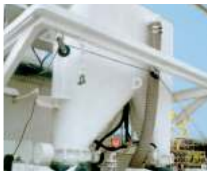
Cement and water weighing system
